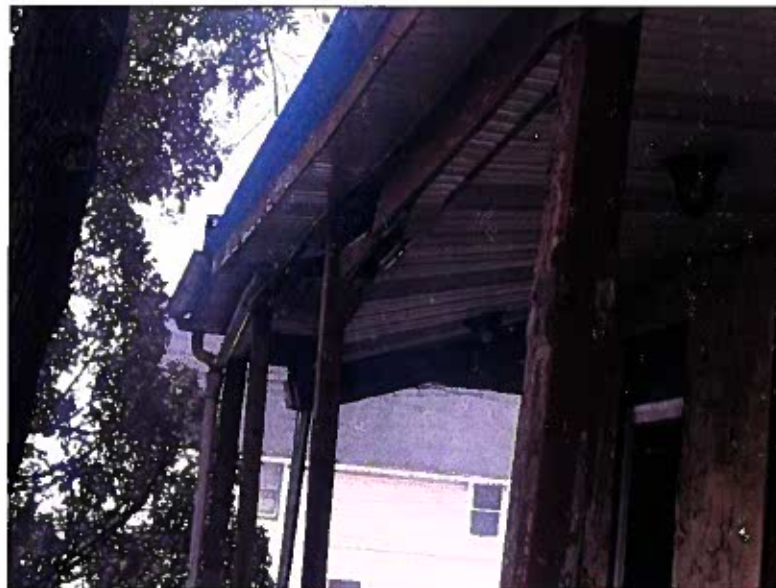
(Photographs of structural damage to front porch. Taken by Dublin Borough Code Enforcement (Ex A).)
