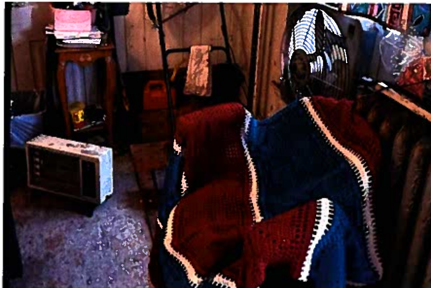
(Photograph of electric space heater in common area and nonfunctional radiator covered with tenant belongings. Taken by Detective John Agnew.)
